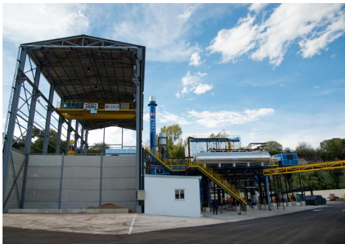
Left: LSolé boiler for Paper Mill industry in Spain
